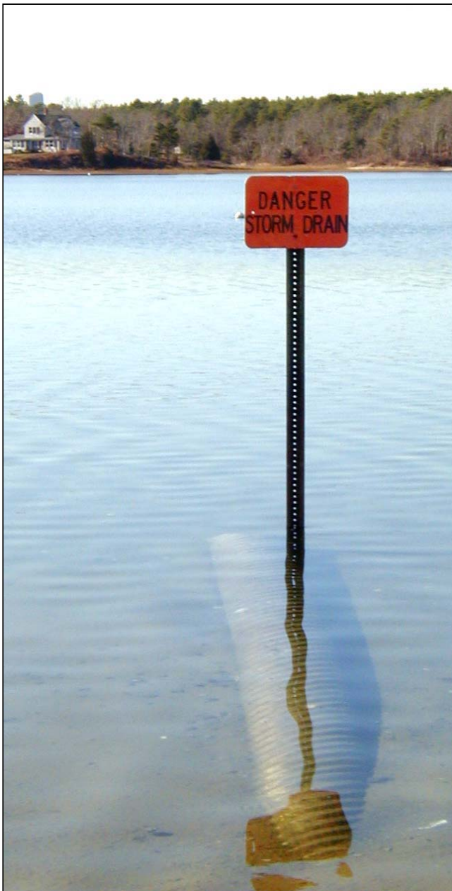
Figure 46. A stormwater discharge pipe in Onset Bay.
