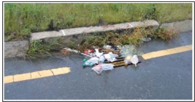
Figure 88. Litter accumulating on a storm drain grate.
